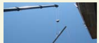
The beam gets lifted to its final resting place atop the new museum.
